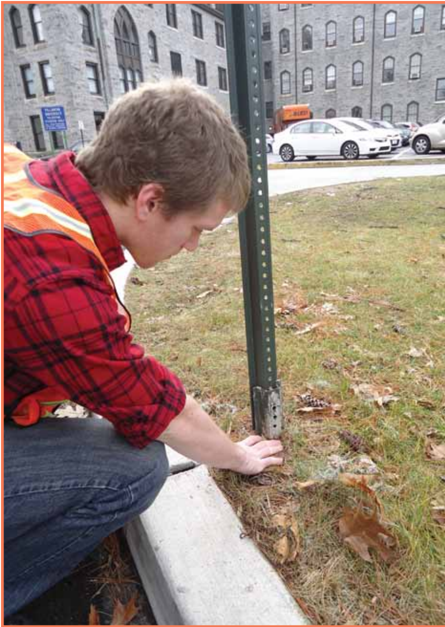
This student is inspecting a breakaway device mounted on a regulatory signpost to check for compliance with MUTCD requirements.
