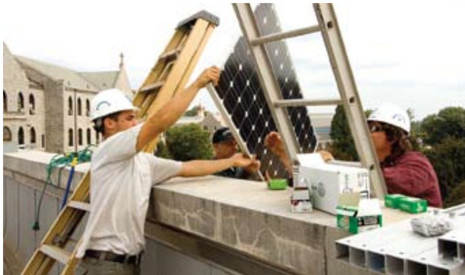
In 2007, technicians mounted 24 solar panels on the south roof of CEER. The installation was the culmination of solar-energy research carried out by graduate engineering students under the guidance of Pritpal Singh, Ph.D., chair of Electrical and Computer Engineering. The College has continued to play a leading role in helping the University create a carbon-neutral campus.
