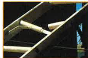
Loose, missing or damaged rungs
