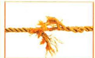
Damaged rope on extension ladder
