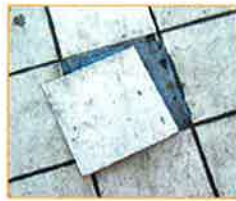
Loose tiles, uneven floors, cracks
