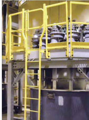
Raised platform with protected guardrail.
