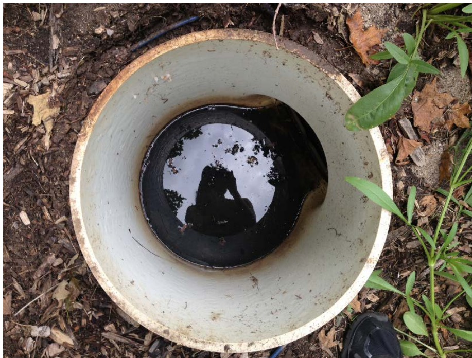
Figure 3.9 The overflow PVC riser, volumetric weir, and discharge pipe (photo credit Villanova Urban Stormwater Partnership). The volumetric weir is located in the discharge pipe that is connected to the overflow riser
