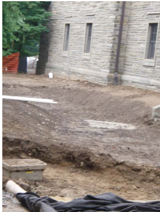
Figure 3.4 Construction of the FRGR at Fedigan Hall (photograph courtesy of Villanova Urban Stormwater Partnership)
