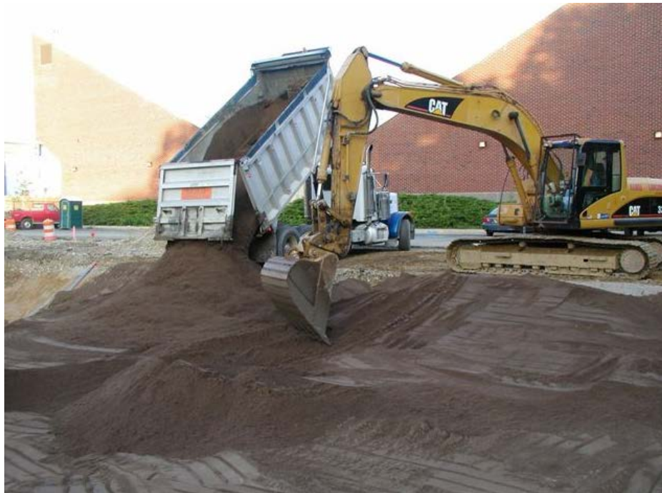
Figure 3.29 Placement of engineered media during construction of the PTI (photograph courtesy of Villanova Urban Stormwater Partnership)
