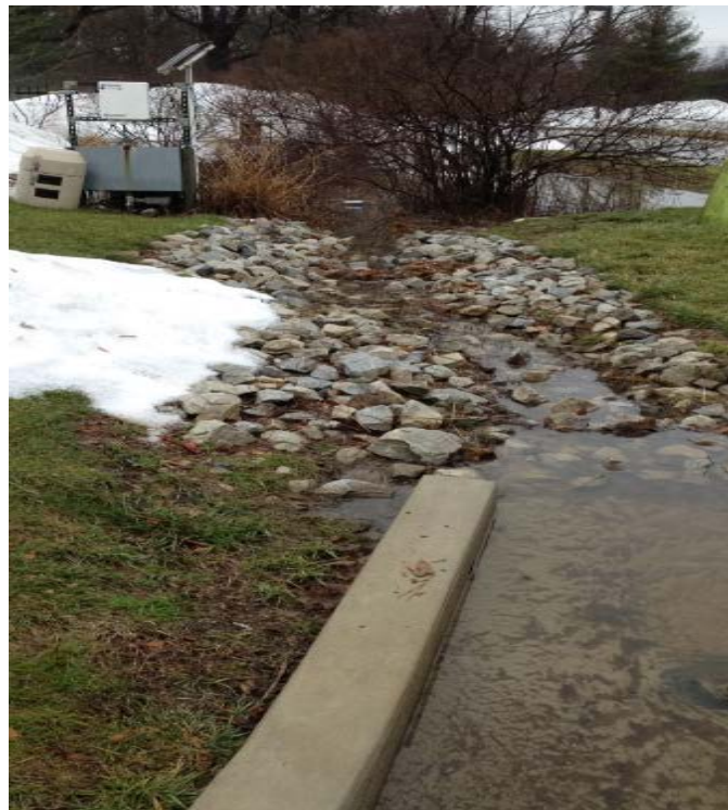
Figure 3.57 The inlet channel leading into the BTI (photograph courtesy of Villanova Urban Stormwater Partnership)
