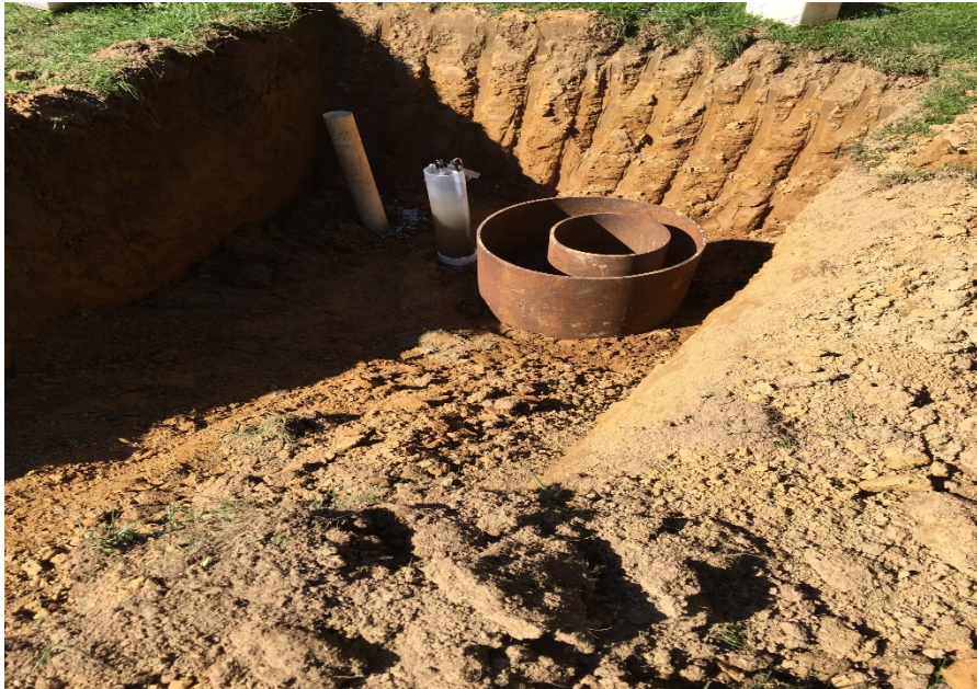
Figure 6.9 Infiltration testing being conducted in a test pit at the Upper Moreland site
