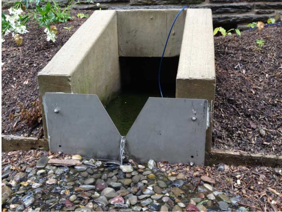
Figure 3.8 A concrete inlet box with a V-notch weir at Fedigan Hall (photograph courtesy of Villanova Urban Stormwater Partnership)
