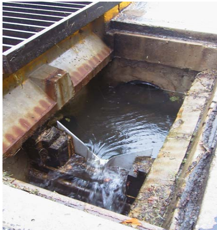
Figure 3.58 The outlet box and weir at the BTI (photograph courtesy of Villanova Urban Stormwater Partnership)
