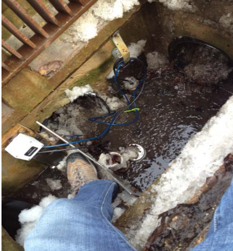
Figure 3.60 Frozen conditions in the outlet box at the BTI (photograph courtesy of Villanova Urban Stormwater Partnership)
