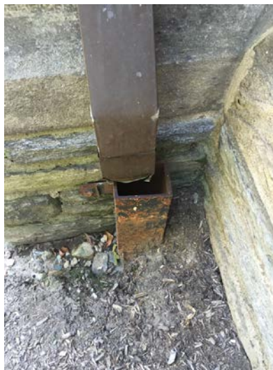
Figure 3.16 A damaged downspout at Fedigan Hall (photograph courtesy of Villanova Urban Stormwater Partnership)
