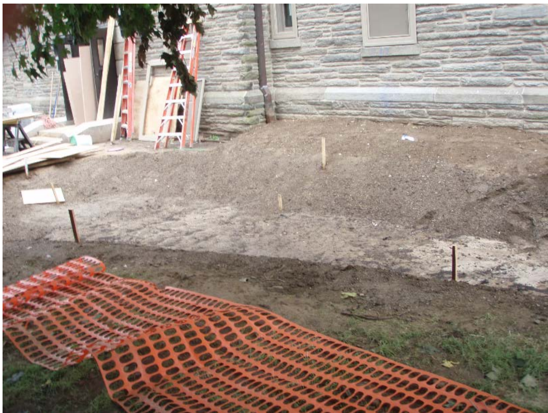
Figure 3.2 Construction of the FRGI at Fedigan Hall (photograph courtesy of Villanova Urban Stormwater Partnership).
