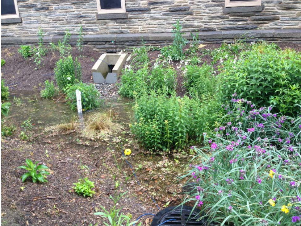
Figure 3.5 The completed FRGR at Fedigan Hall (photograph courtesy of Villanova Urban Stormwater Partnership)
