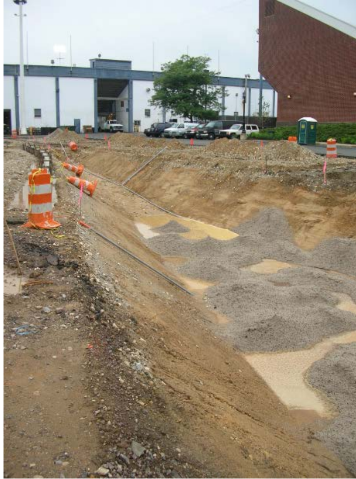
Figure 3.35 The PTI ponded during construction (photograph courtesy of Villanova Urban Stormwater Partnership)
