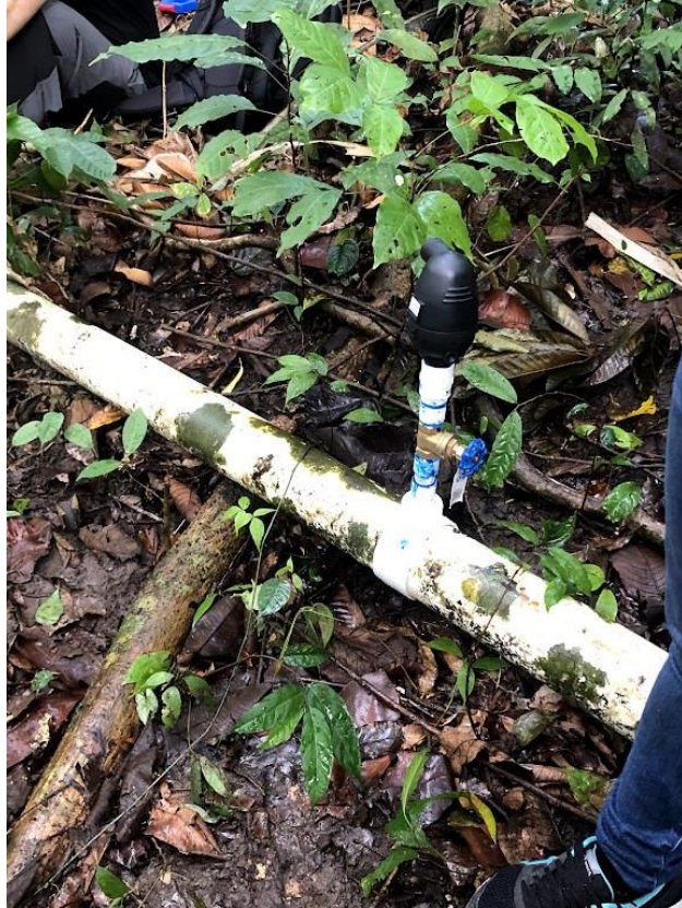
12 - Air release valve installed on the water system.
