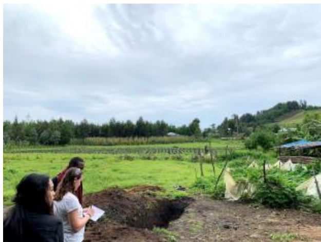
23 - Tanzania: Photo of myself assessing a site being considered for the implementation of a biogas reactor.
