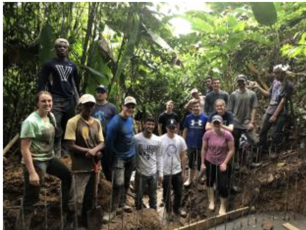
25 - Nicaragua: Photo of the Villanovan team with construction workers helping to build the water intake tank and distribution system.
