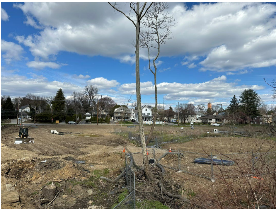
Figure 4. Photo of the West Wayne Preserve under construction. After the regrading work to provide additional storage, it will be filled with high quality wooded wetland vegetation.
